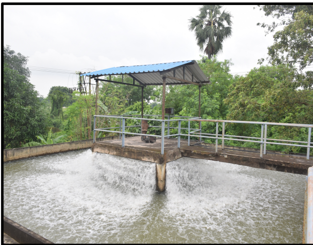
Flocculator at Balram STP
