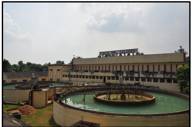
Clarifier at IWSS, Talcher
