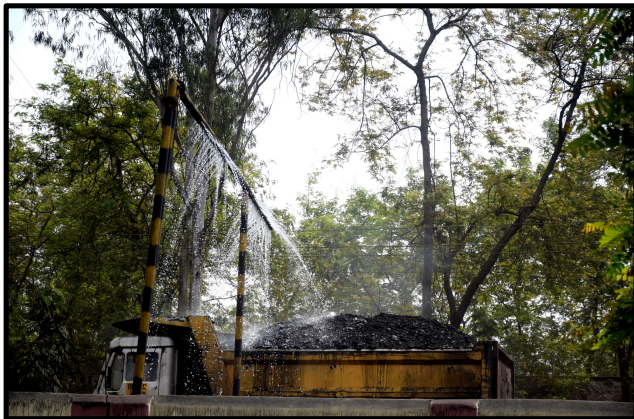
Instant Shower system at Lakhapur OCP
