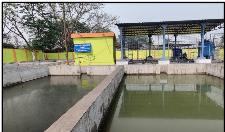
Secondary settling tank, at ETP Jagannath OCP
